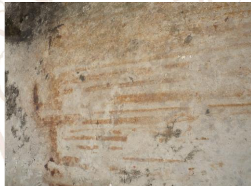
Rust marks on garage floor
